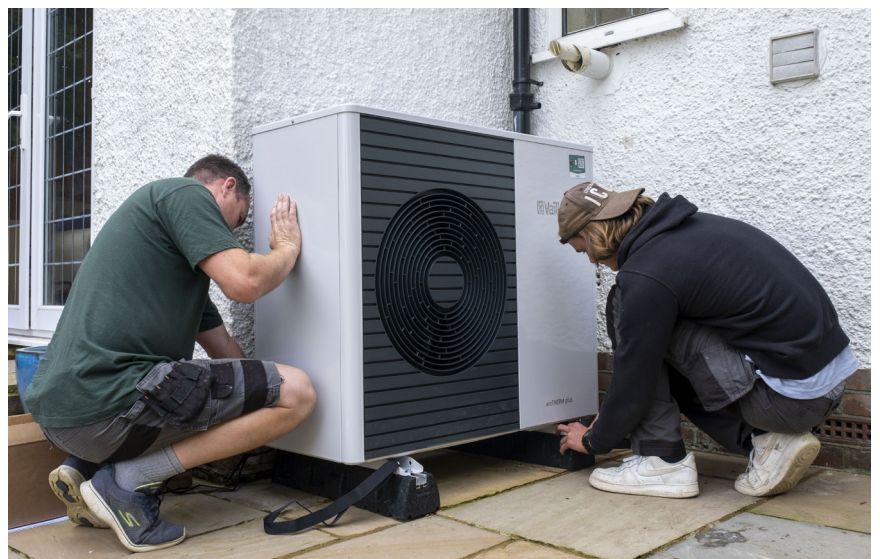
In Folkestone, a town in England, installers set up a heat pump for a house built in the 1930s. Image: Andrew Aitchison / In pictures via Getty Images
